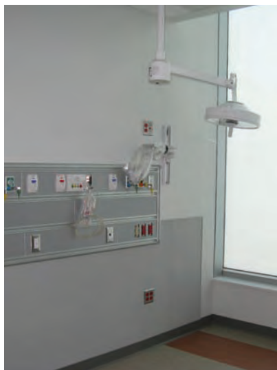
Larger treatment rooms will feature removable cabinetry to allow for surge capacity.
